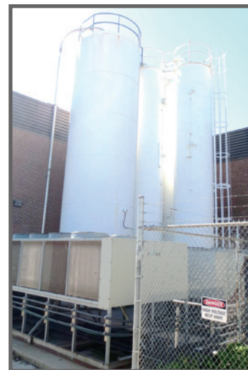
TRANE/CONAIR CHILLERS & SILOS
